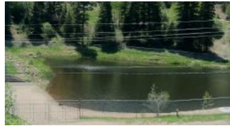
King Murphy Augmentation Pond is located on Witter Gulch in Clear Creek County and serves as a sediment catchment basin for the drainage system. Sediment deposition from 2013 flooding filled the basin. The county completed a restoration effort to repair and upgrade this catch basin and augmentation pond.
